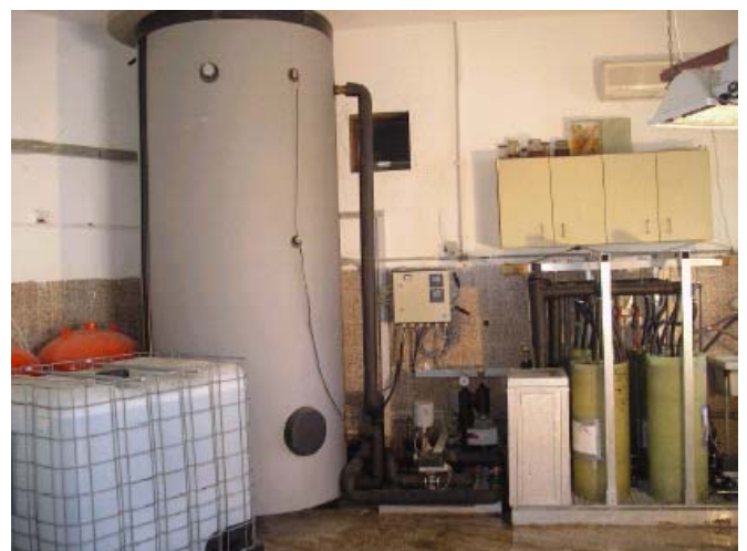
Fig.5 Picture of the desalination unit
