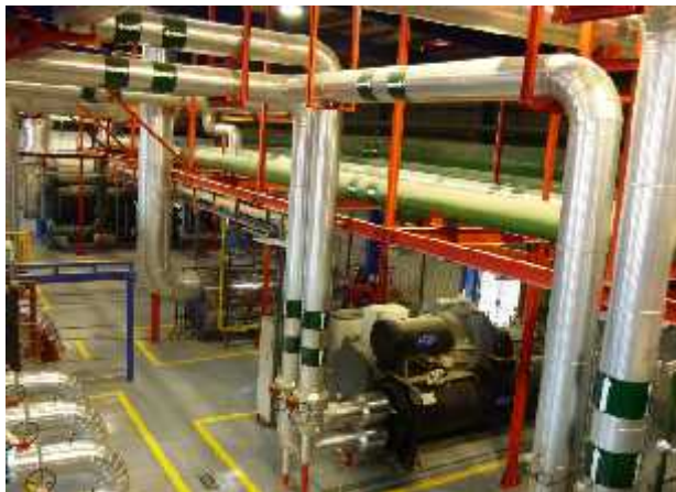
Figure 7 Internal view of the ST-4 energy plant
