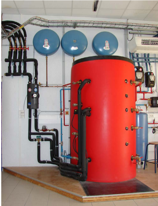
Fig. 3: Storage tank and its functional scheme.
