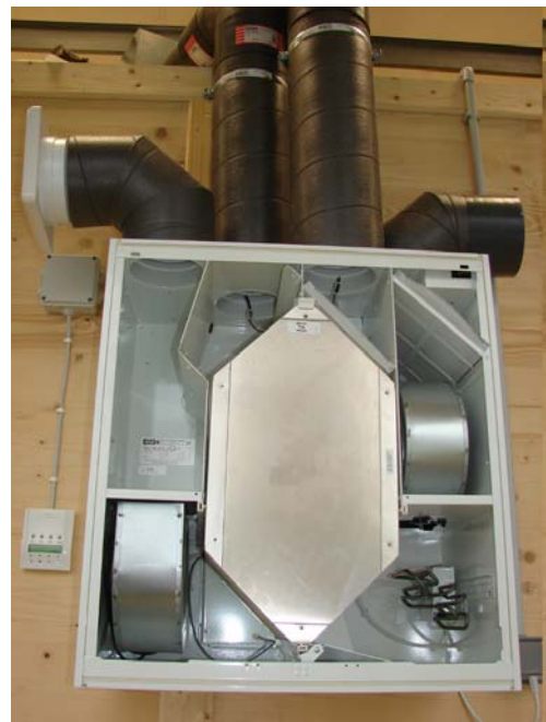
Fig. 11: Heat recovery ventilation
