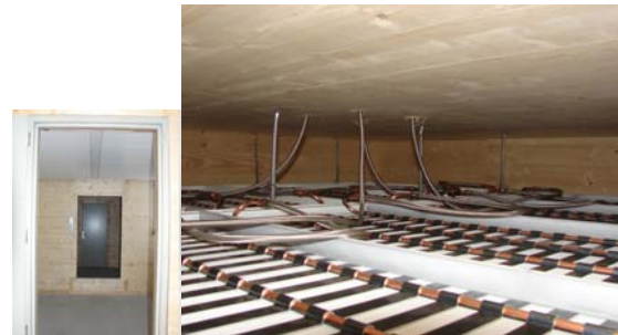
Fig. 10: The cold chamber (a) Inside the room; (b) Chilled ceiling
